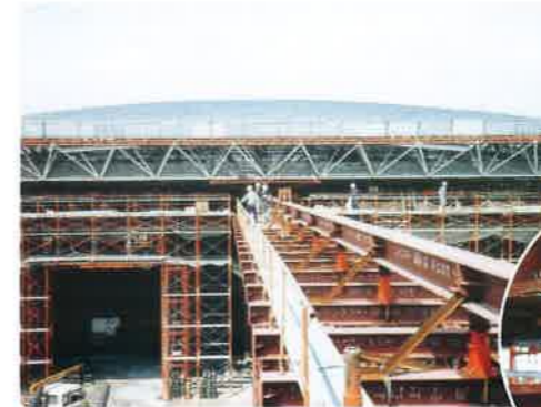
大型屋根スライド工法 (NEWS 0166) Slide method of large roof construction
