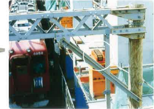
橋梁架台の引き込み (NEWS 0153) Lead-in work of a bridge girder mount
